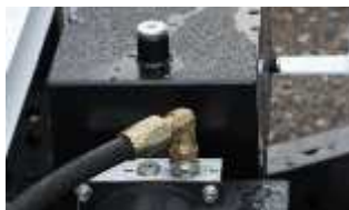
12 volt Tipping unit upgrade
